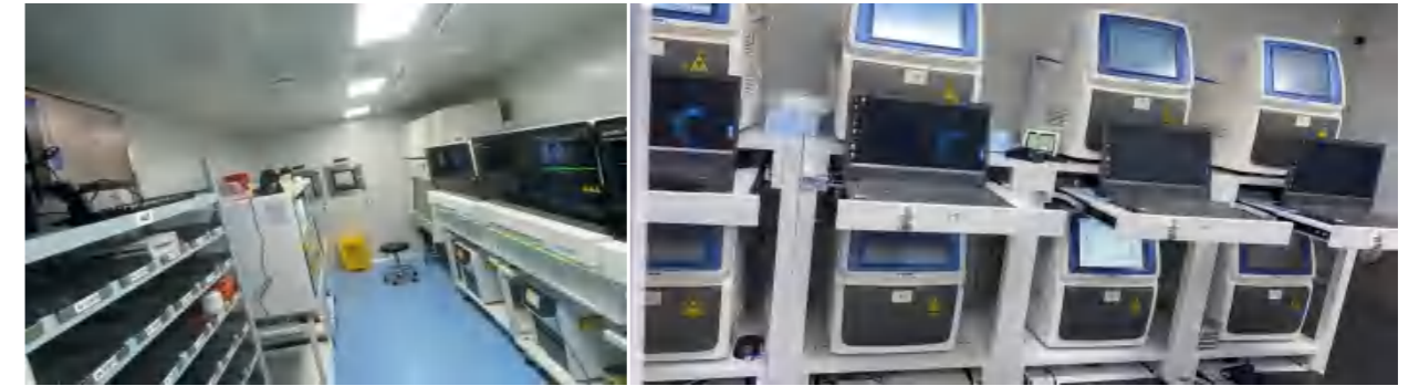
Beijing Children's Hospital Landing container mobile laboratory (two cabins). Daily testing capability can be up to 10,000 tubes per day in each cabin.
